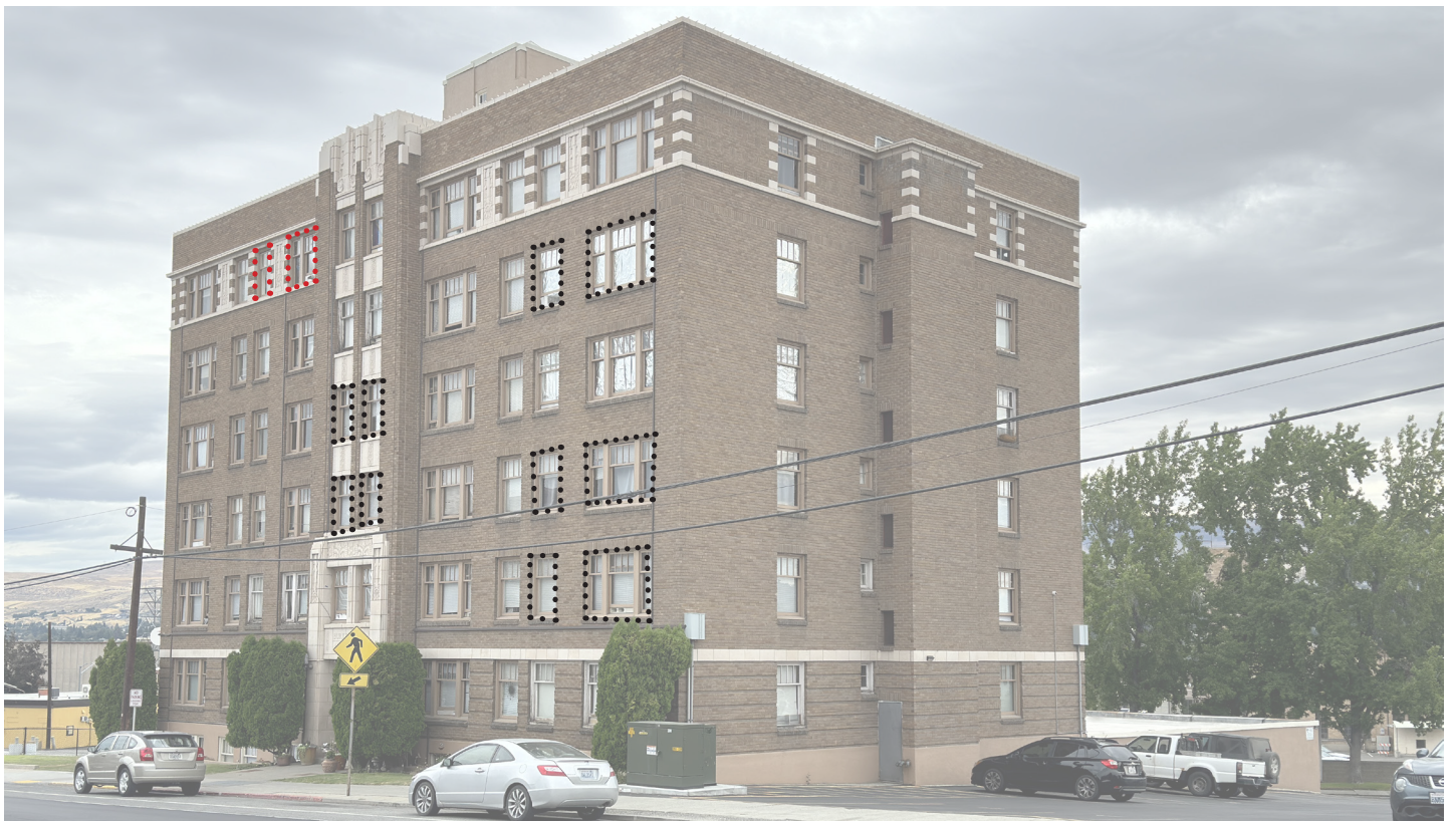
IMAGE 4. After: 2024, exterior walls, front northwest corner. Repaired windows, black dots outline work completed in 2022; red dots outline work completed in 2024.
