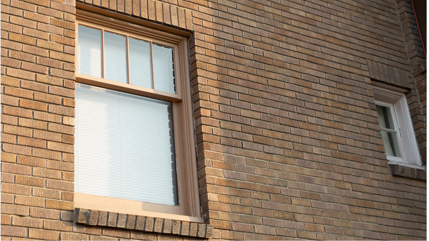
IMAGE 9. After: 2022, south facade, west side, second story showing a typical repaired window.
