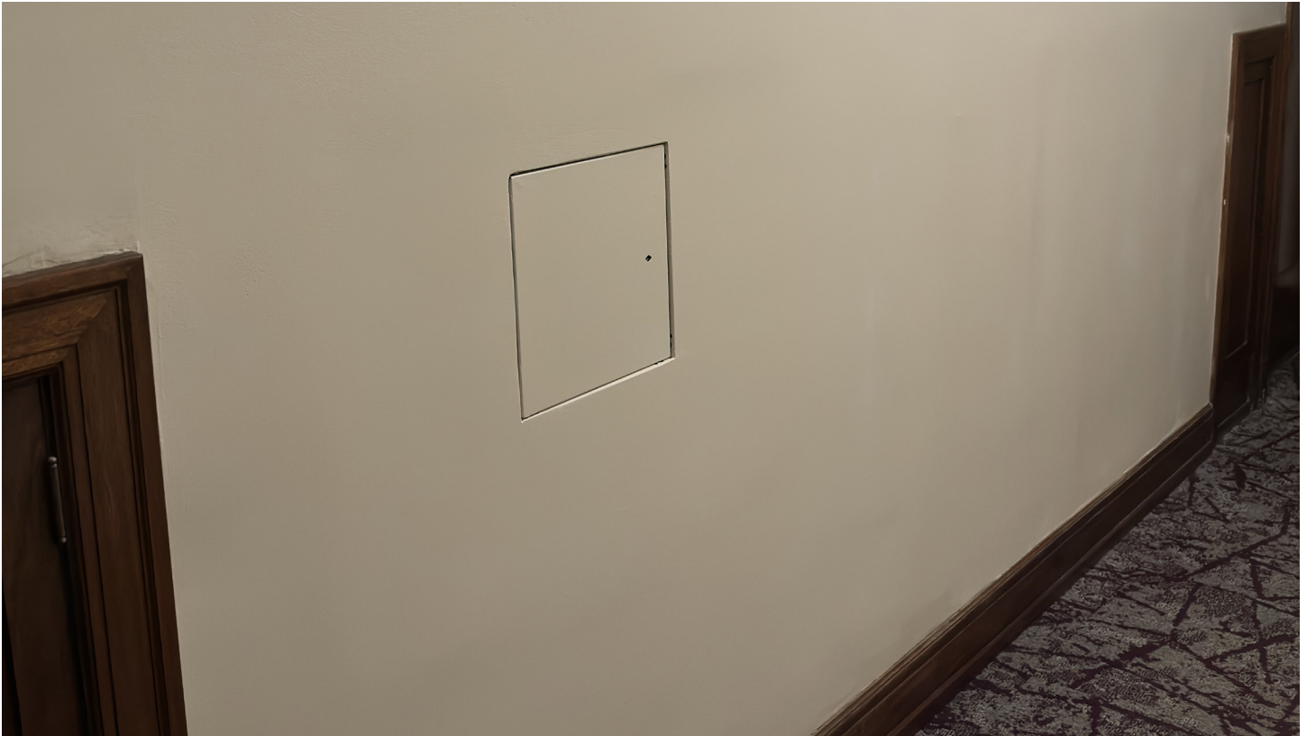
IMAGE 36. After: 2024, first floor, showing a typical new metal access panel within the hallway for plumbing valve access allowing floor sections to be closed off for repairs without having to shut down the full building.
