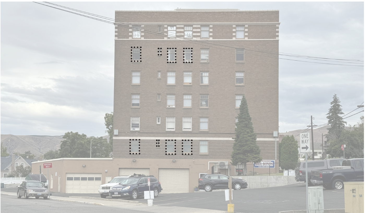
IMAGE 6. After: 2024, exterior walls, north facade. Repaired windows, black dots outline work completed in 2022. No window repairs were completed on this facade in 2024.
