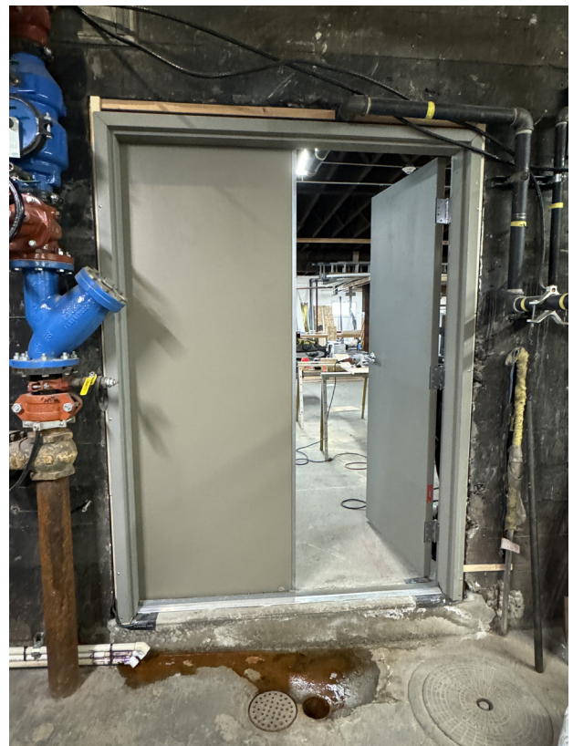
IMAGE 44. After: 2024, basement, boiler room, east wall, showing added doorway enabling water heater installation.
