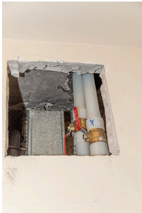
IMAGE 37. Before: 2022, sixth floor, looking southwest showing the valves within a typical new metal access panel location.
