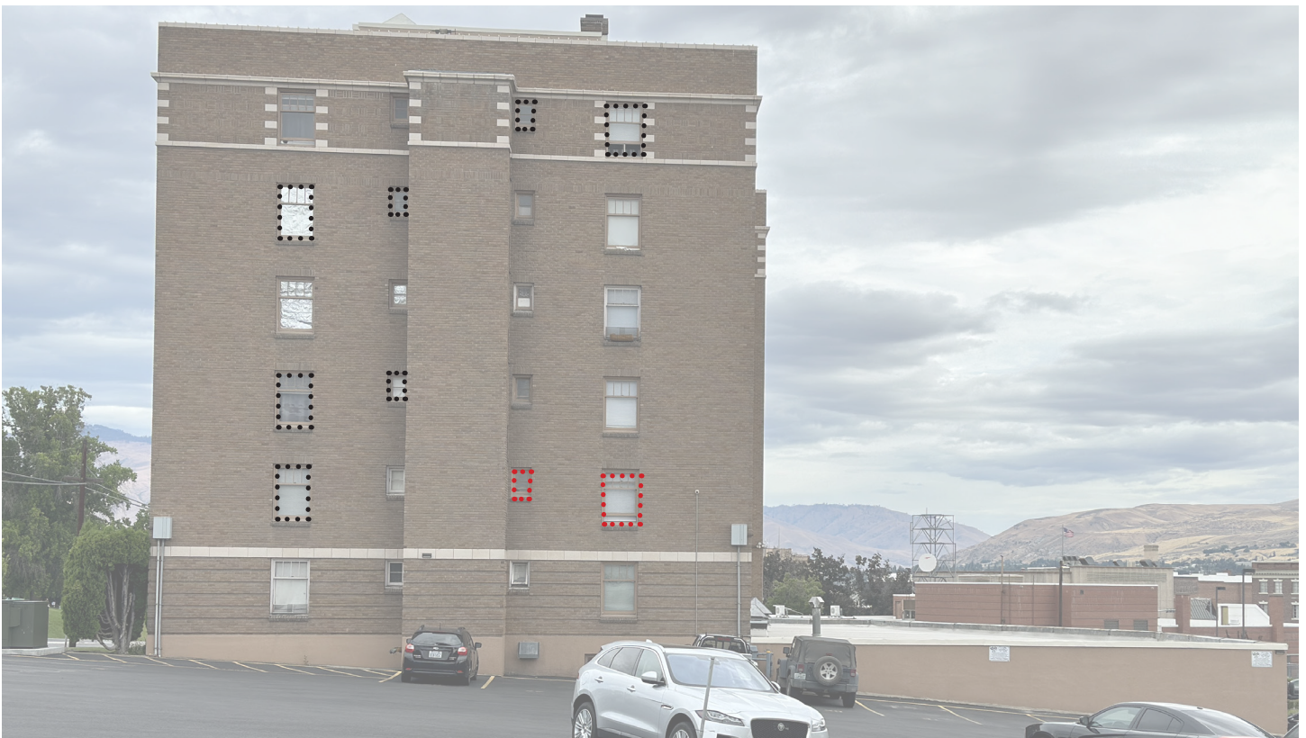
IMAGE 2. After: 2024, site, south facade, looking north across Yakima Street. Repaired windows, black dots outline work completed in 2022; red dots outline work completed in 2024.
