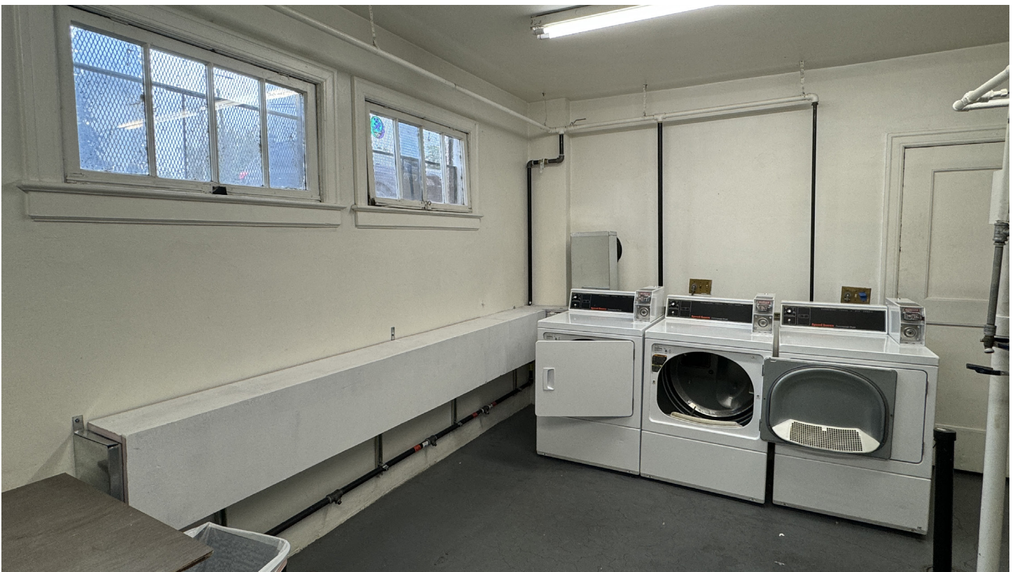
IMAGE 41. After: 2024, basement, laundry room, looking southwest showing new drier ducting installed along the south wall in order to relocate the driers to this wall and add an additional drier.
