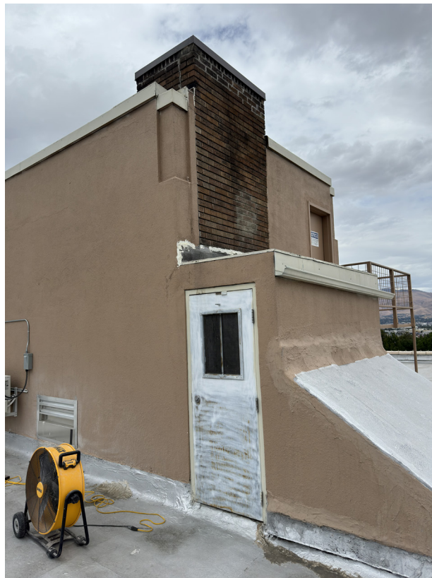
IMAGE 39. After: 2024, penthouse, south east corner, showing the chimney repairs and sheet metal cap.
