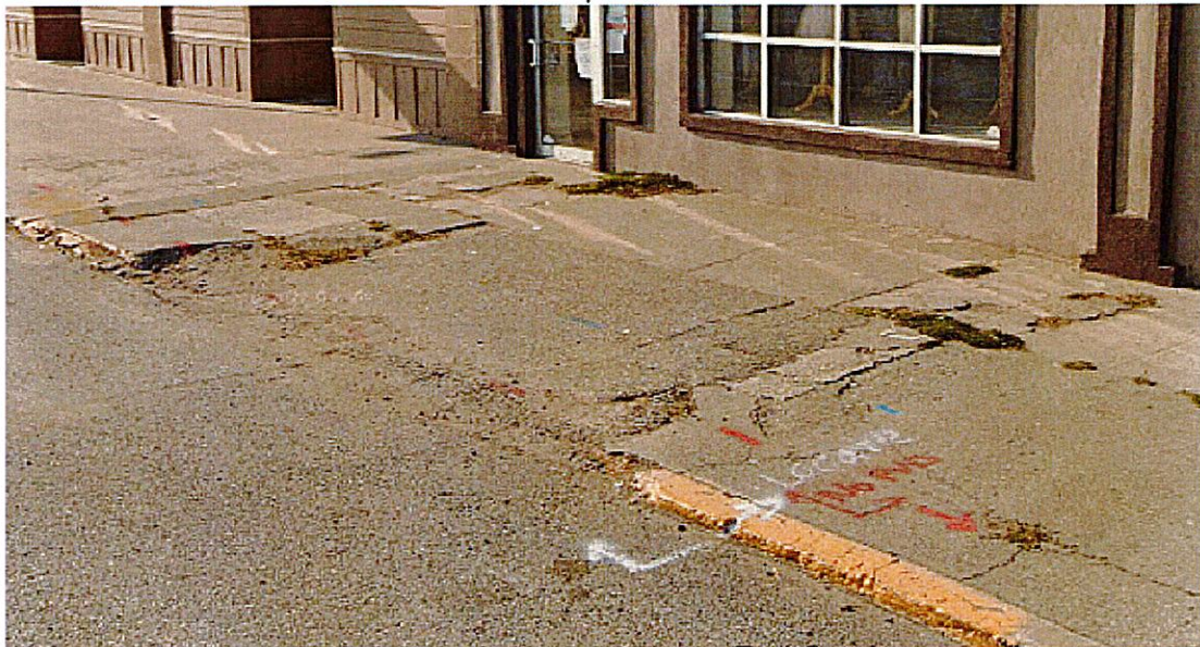
804 South Wenatchee sidewalk before replacement
