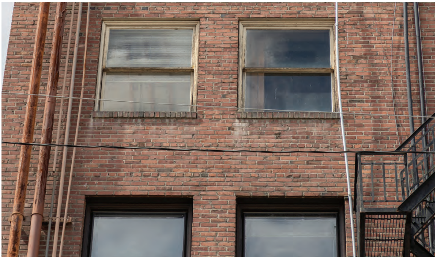
Fig. 16. East facade, south portion, third (partial) and fourth story windows showing existing conditions.
