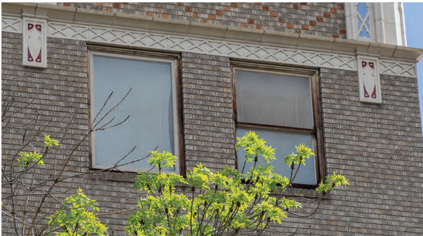
Fig. 5. West facade, fourth story, south windows, showing a replacement window and wood window conditions.
