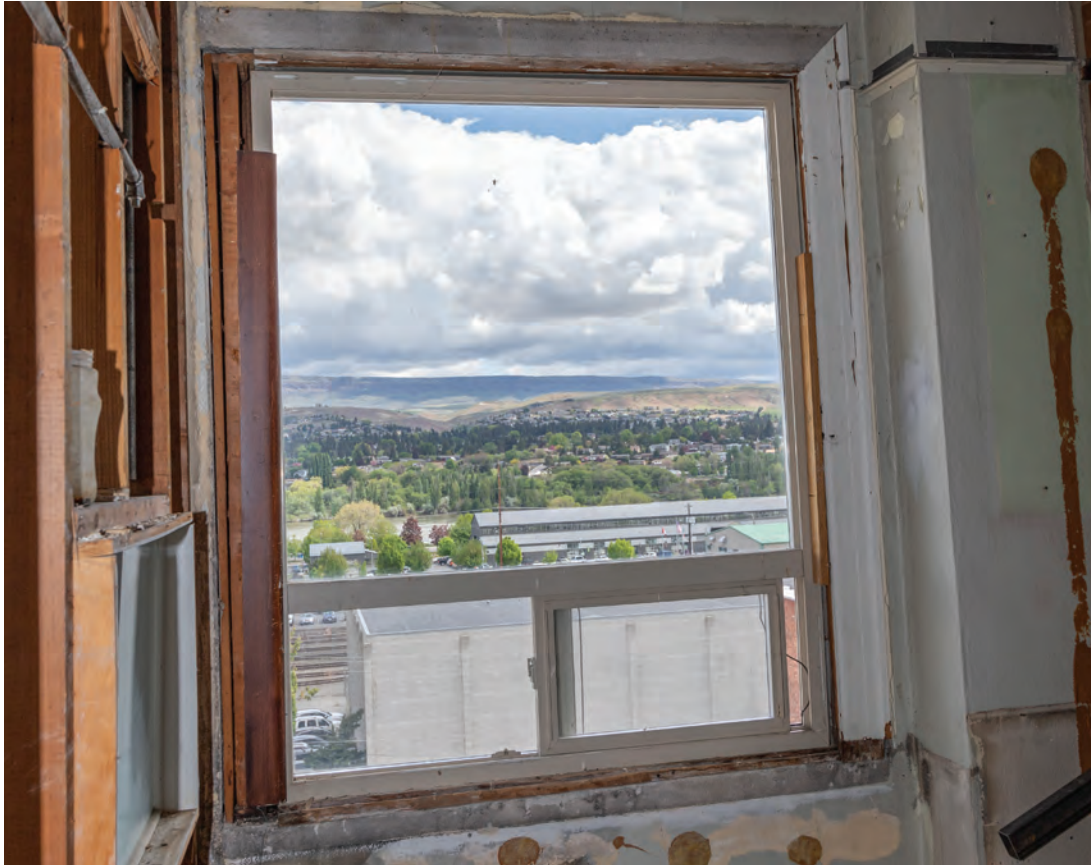
Fig. 18. East facade, north portion, fourth floor, showing remnant trim at a replacement window.
