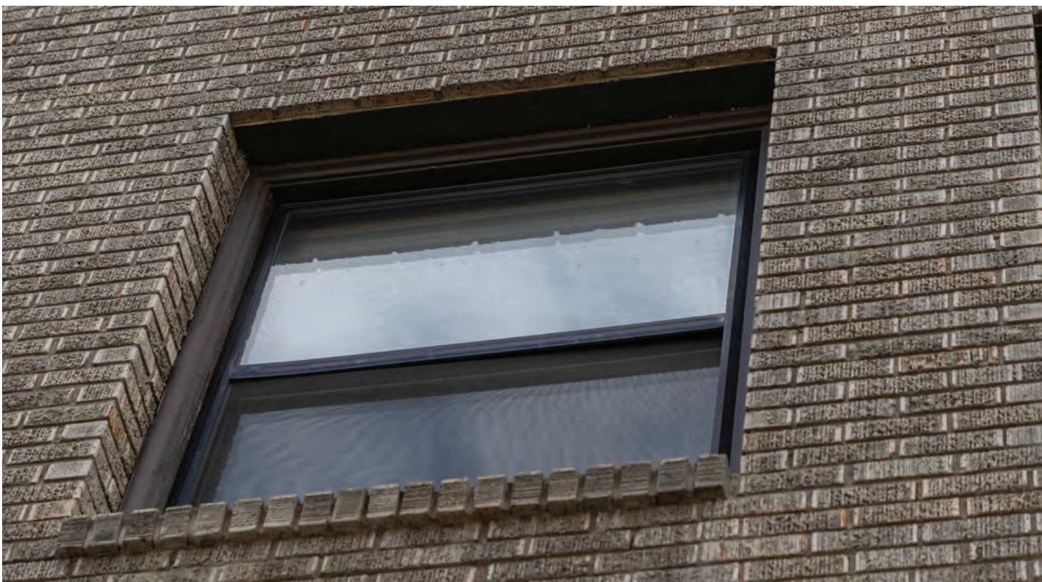
Fig. 10. North facade, east portion, third story, showing previous replacement window conditions.
