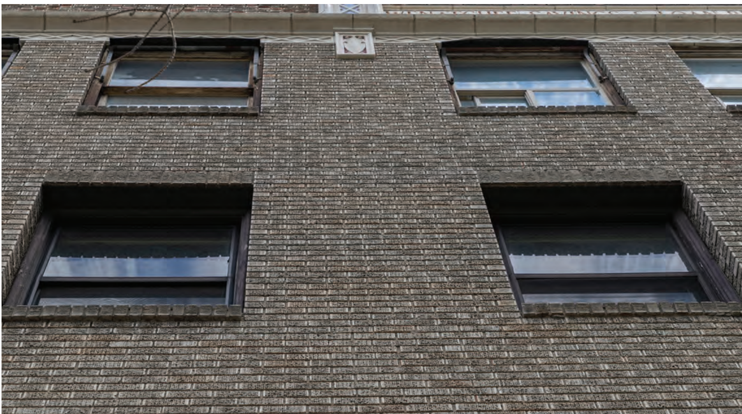
Fig. 7. West facade, looking up from the sidewalk showing window headers and window conditions.
