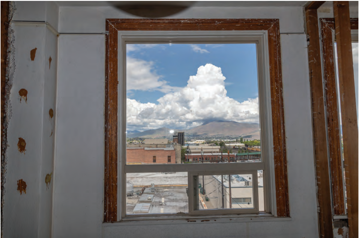
Fig. 14. North facade, fourth floor, view showing a previous replacement window, window trim painted with some areas partially stripped, and a missing apron.
