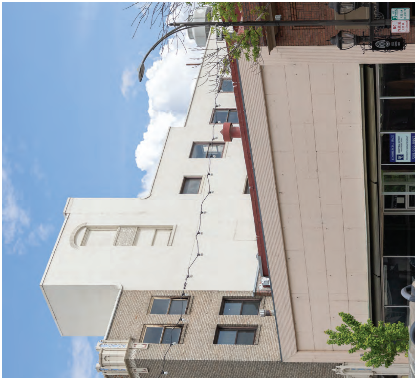
Fig. 20. South facade, west and central portions (above left) and east portion (above right) showing typical conditions.
