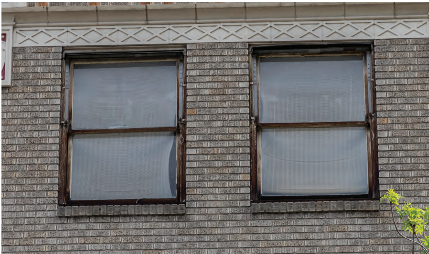
Fig. 4. West facade, fourth story, north windows, showing wood window conditions.
