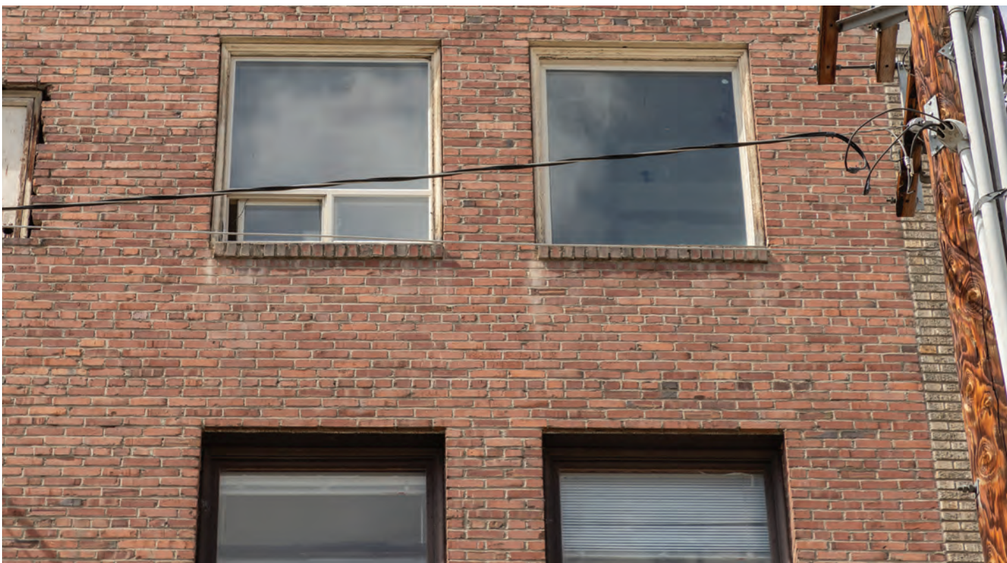
Fig. 17. East facade, north portion, third (partial) and fourth story windows showing existing conditions.
