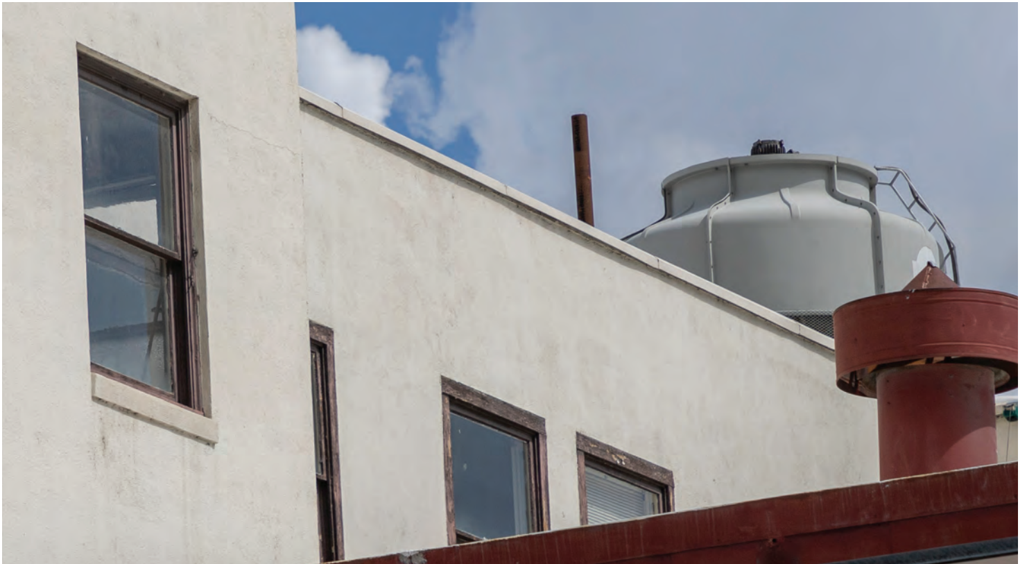
Fig. 19. South facade, west portion, fourth story, showing window conditions.
