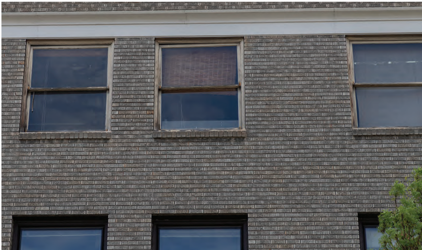
Fig. 9. North facade, east portion, fourth story windows showing wood window conditions.
