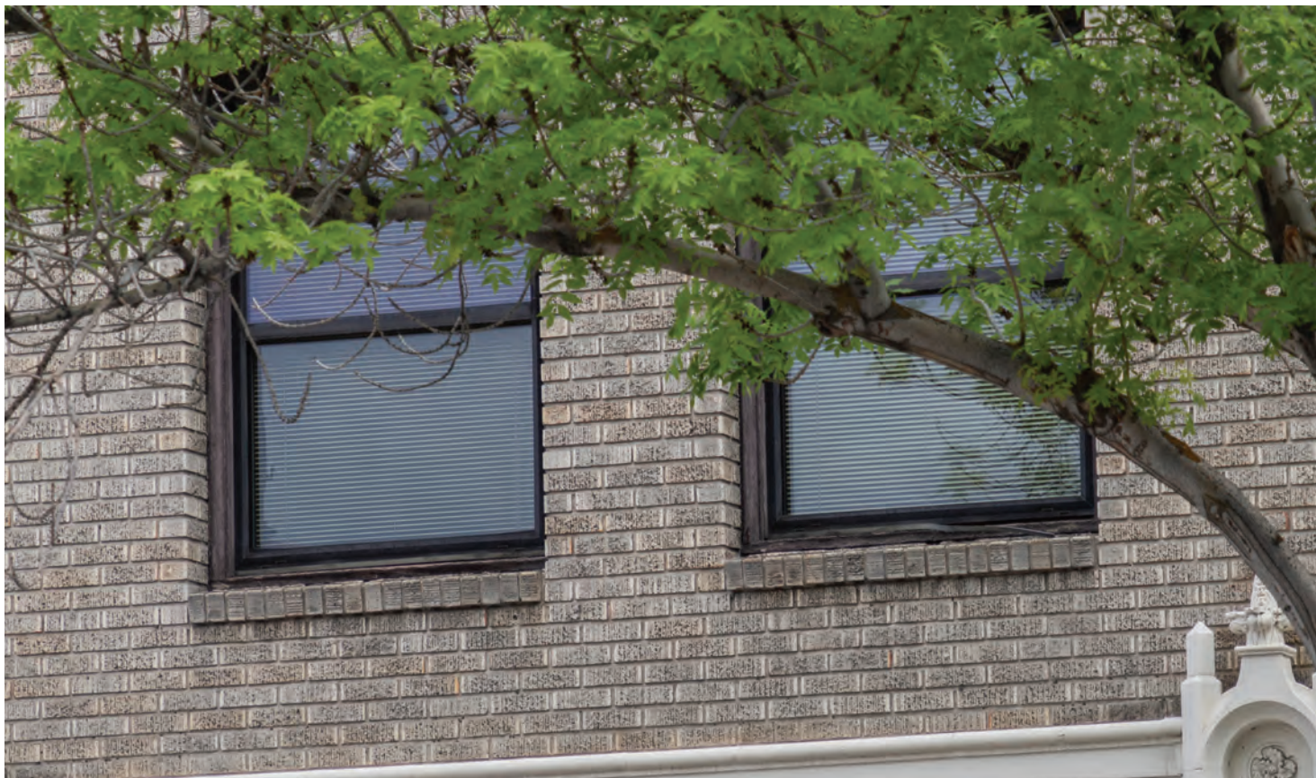
Fig. 6. West facade, second story, north windows, showing conditions of previous replacement windows.
