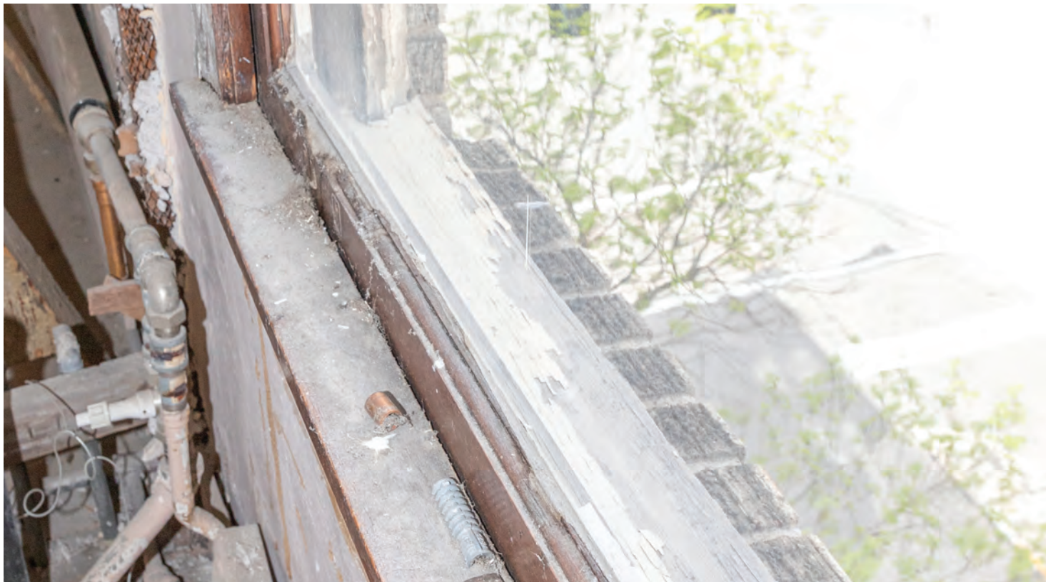
Fig. 12. North facade, fourth floor, interior detail showing exterior sill configuration and condition.
