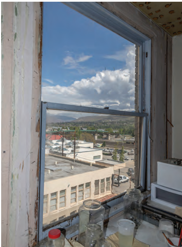
Fig. 11. North facade, fourth floor, west portion, interior detail showing typical configuration and conditions.
