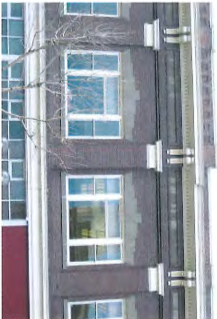
View o Second story cornice and window details Photography Neg. No (Roll No./Frame No.): Nov06-032 taken 11/14/2006 Comments:
