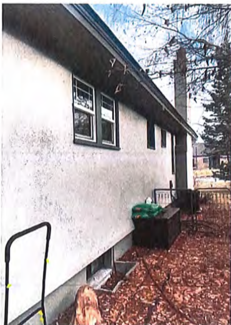
Photo from the NW corner of the house looking toward Idaho St. Another egress window will be added here where the existing window is seen along the ground. Just like the other egress window described above, you may be able to see the work being done on this window but the final product will not necessarily be seen from the sidewalk.
