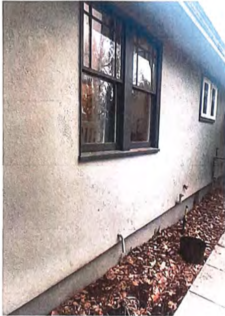
Photo of the SE corner of the front of the house. An egress window will be added here. The window will be placed under the kitchen windows which in this photo are white. Although you will be able to see the work being done, the final product will not necessarily be seen from the sidewalk.
