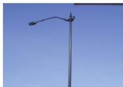
Street lighting / Alumbrado urbano
