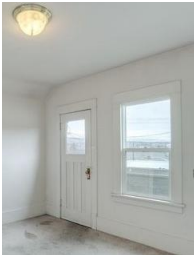
Balcony Door Before
