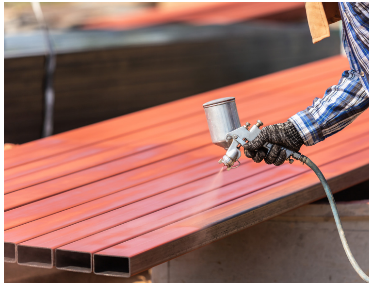
Metals should be painted or coated to prevent corrosion
