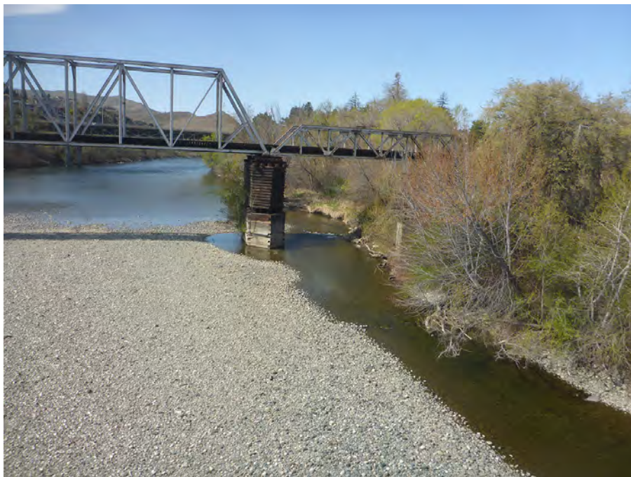
Photograph 10 Wenatchee River Left Bank and Side Channel Upstream of Apple Capital Recreational Loop Trail Bridge
