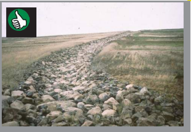
Good example of a rock lined interceptor swale. (Source: Peter Vaughn, A3E Consultants)
