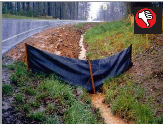
Silt fence is not an approved BMP for use as a check dam.
