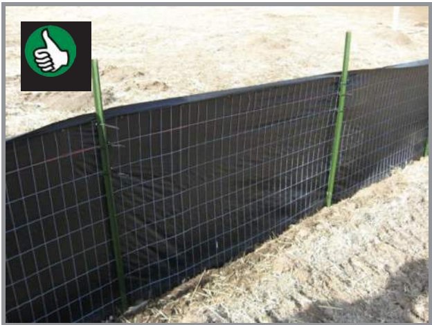
Properly installed silt fence using steel posts and wire mesh backing. (Source: URSCorporation)
