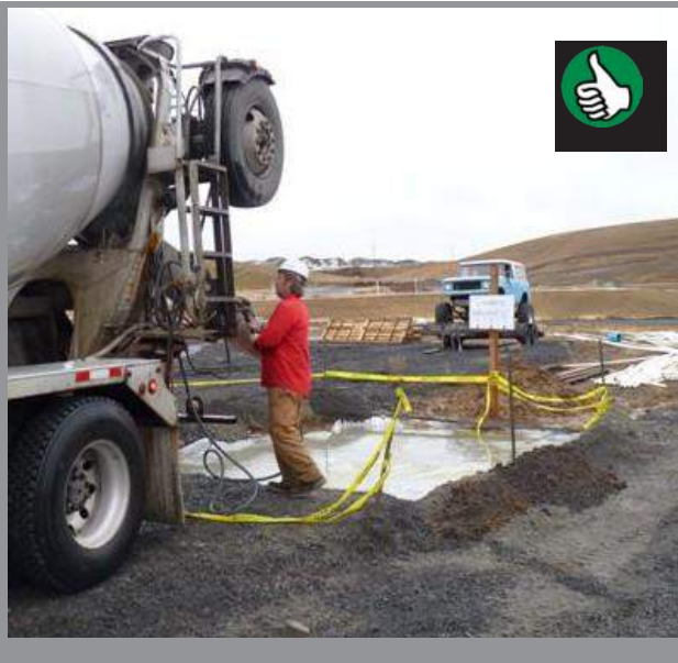
Good example of properly designed concrete washout area. (Source: City of Pullman)
