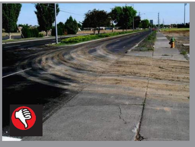
Stabilize or maintain construction exits to prevent trackout. (Source: City of Moses Lake)
