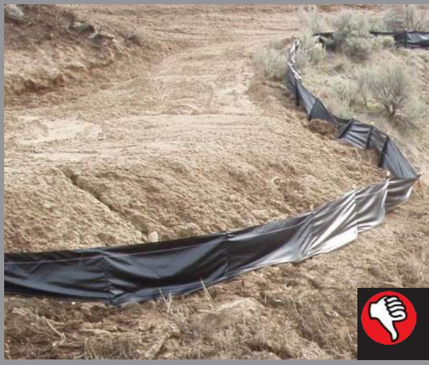
Silt fence is installed backwards; posts should be on downhill side. (Source: City of Wenatchee)
