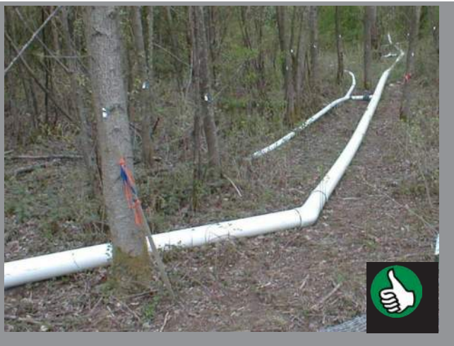
Six inch pipe draining a sediment pond. The six inch pipe drains into four inch perforated pipe which allow the sediment laden water to percolate through the duff and soil. (Source: WSDOT)
