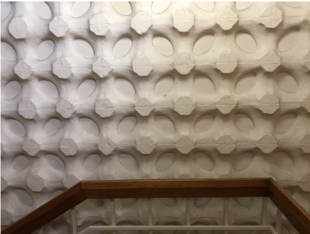
Detail of concrete wall in stairway from first floor entrance off Orondo St. side of building to main floor.
