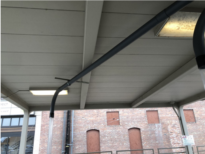
Pneumatic tubes, lighting under carport
