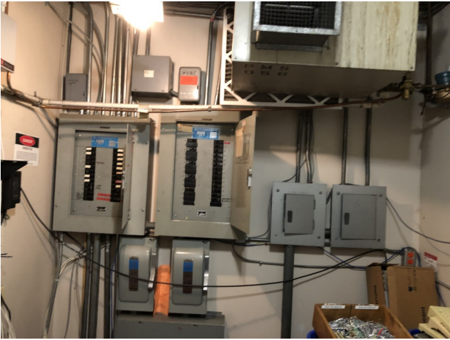
Interior, electrical room
