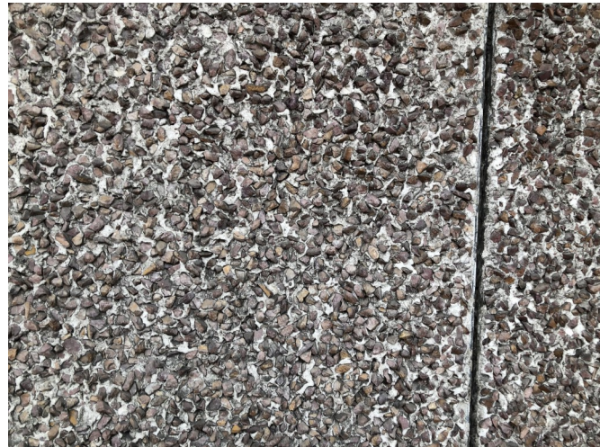
Aggregate material on walls
