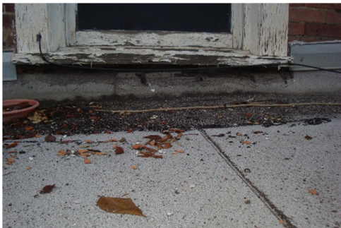
Rotting wood sill near roof (south)
