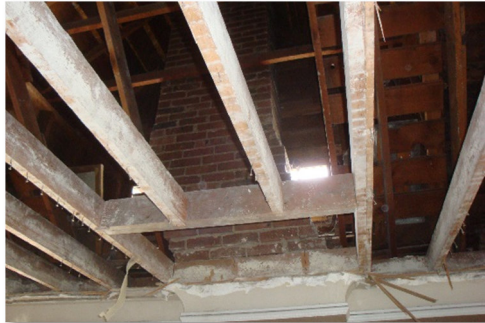
Masonry chimney obstructing dormer windows
