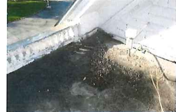
Rebuild this roof
