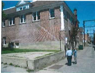
Mineral deposits on brick
