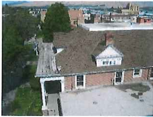
Flat roof areas need repair
