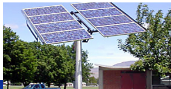
Pioneer Middle School Solar Panels
