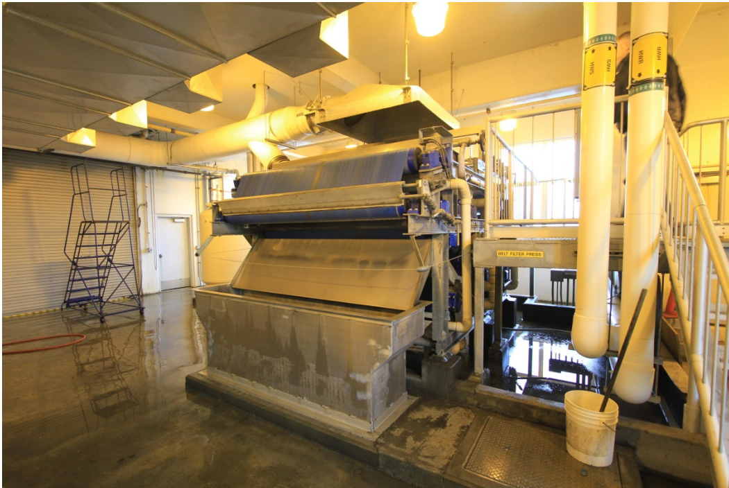
Figure 3-19. Existing Belt Filter Press
