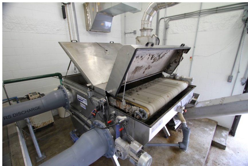
Figure 5-1. Salsnes™ Primary Belt Filter
