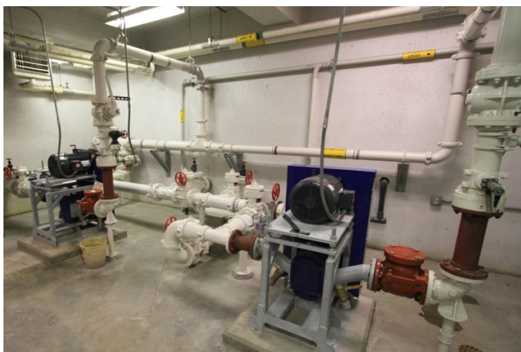
Figure 3-7. Primary Sludge Pump Station
