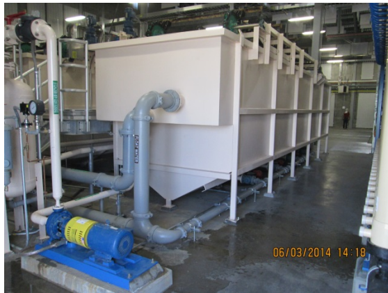
Figure 5-6. Typical DAF Thickener Installation
