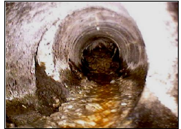
This picture shows the GREASE in the sewer line of a Commercial Kitchen in Wenatchee, WA. The picture was taken in September of 2003.
