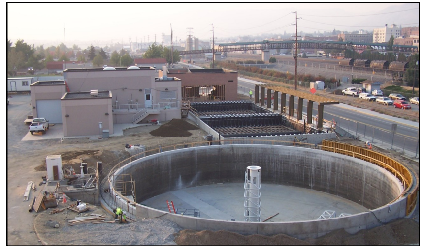
Updates to the primary clarifier
